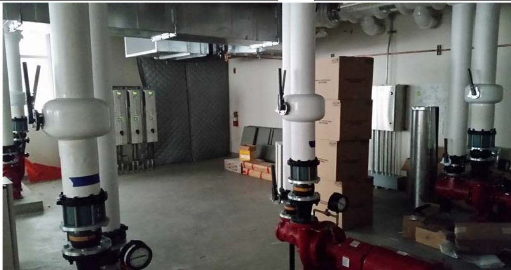
Central Plant geothermal pumps
