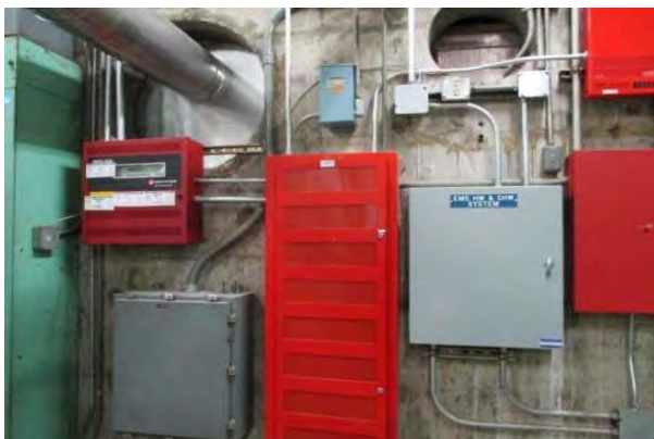
#41: FIRE ALARM CONTROL PANEL, ADDRESSABLE
