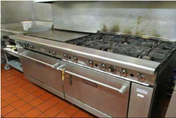
#45: COMMERCIAL KITCHEN, RANGE/OVEN, 6-BURNER W/ GRIDDLE
