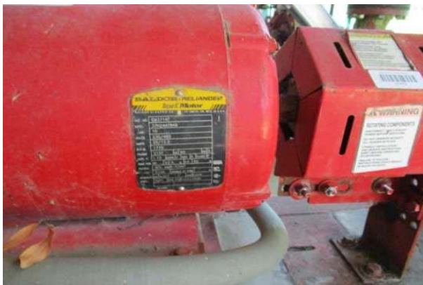
#35: DISTRIBUTION PUMP, CHILLER & CONDENSER WATER
