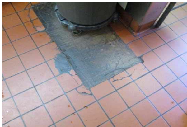
#18: KITCHEN QUARRY TILE, CRACKED AND BROKEN
