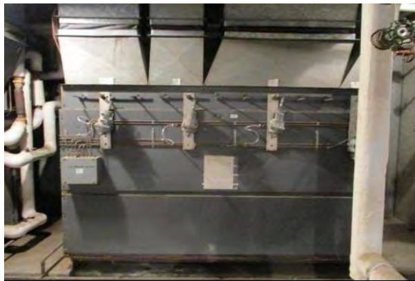
#34: AIR HANDLER, INTERIOR
