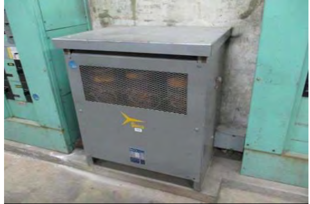
#38: SECONDARY TRANSFORMER, DRY
