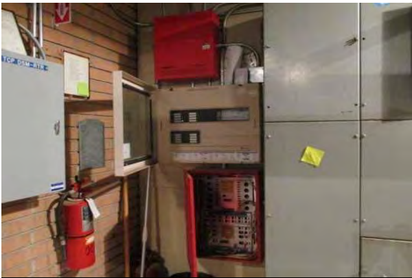
#37: FIRE ALARM CONTROL PANEL
