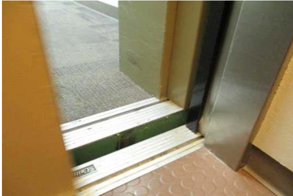
#19: ELEVATOR CONTROLS, DOOR OPENS BEFORE FLOORS ARE LEVEL
