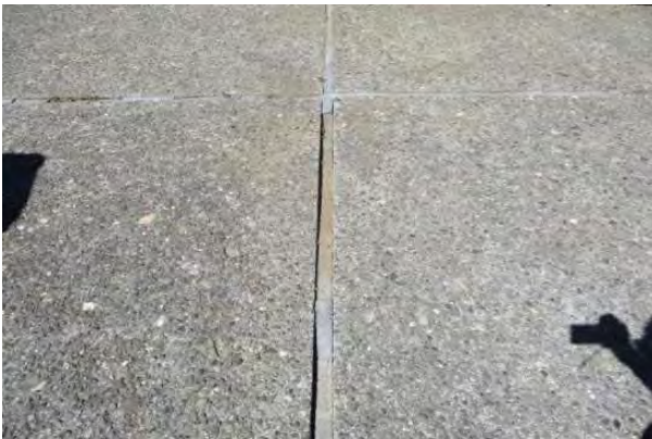
#47: ROTTED WOOD EXPANSION STRIPS
