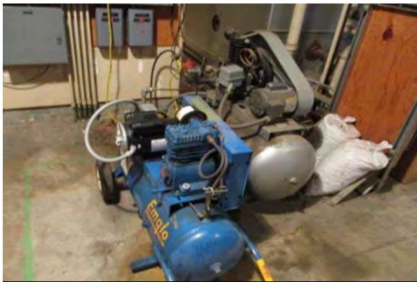
#33: HVAC CONTROLS, PART PNEUMATIC, AIR COMPRESSOR
