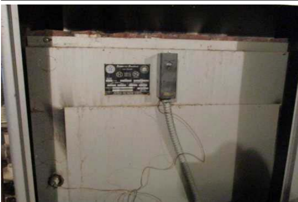
#29: BOILER, GAS, DOMESTIC & HEATING
