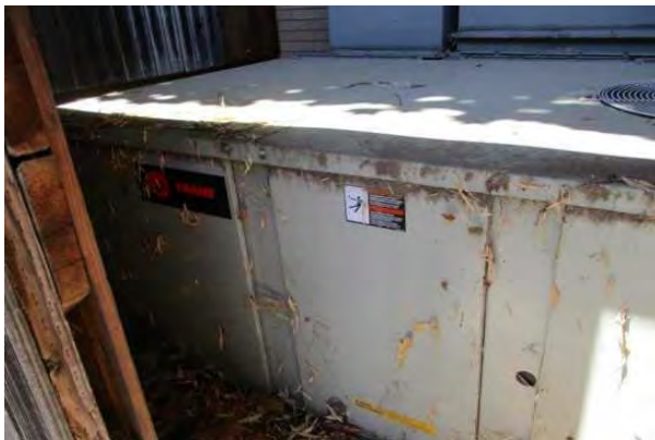
#35: HEAT PUMP, PACKAGED
