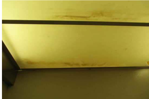
#20: ELEVATOR CAB FINISHES, STANDARD
