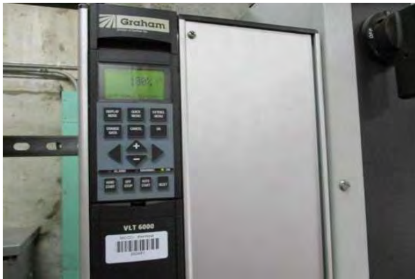
#33: VARIABLE FREQUENCY DRIVE (VFD)
