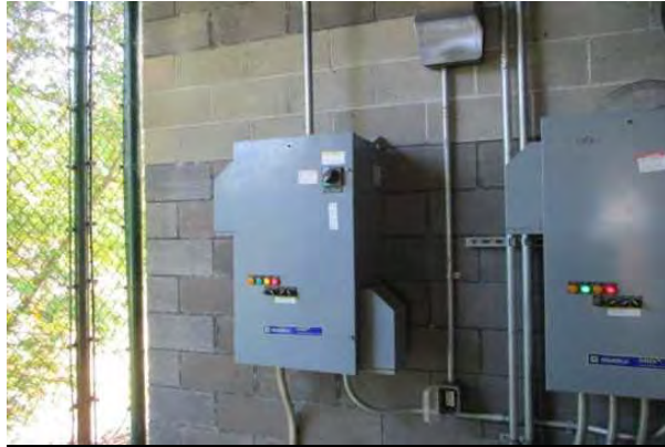
#32: VARIABLE FREQUENCY DRIVE (VFD)
