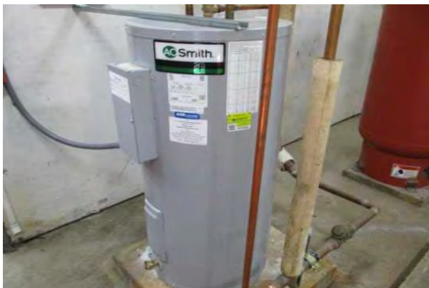
#23: WATER HEATER, ELECTRIC, COMMERCIAL
