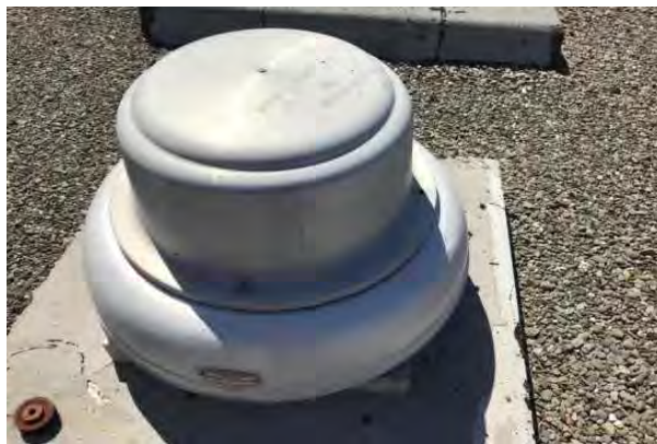
#36: EXHAUST FAN, CENTRIFUGAL
